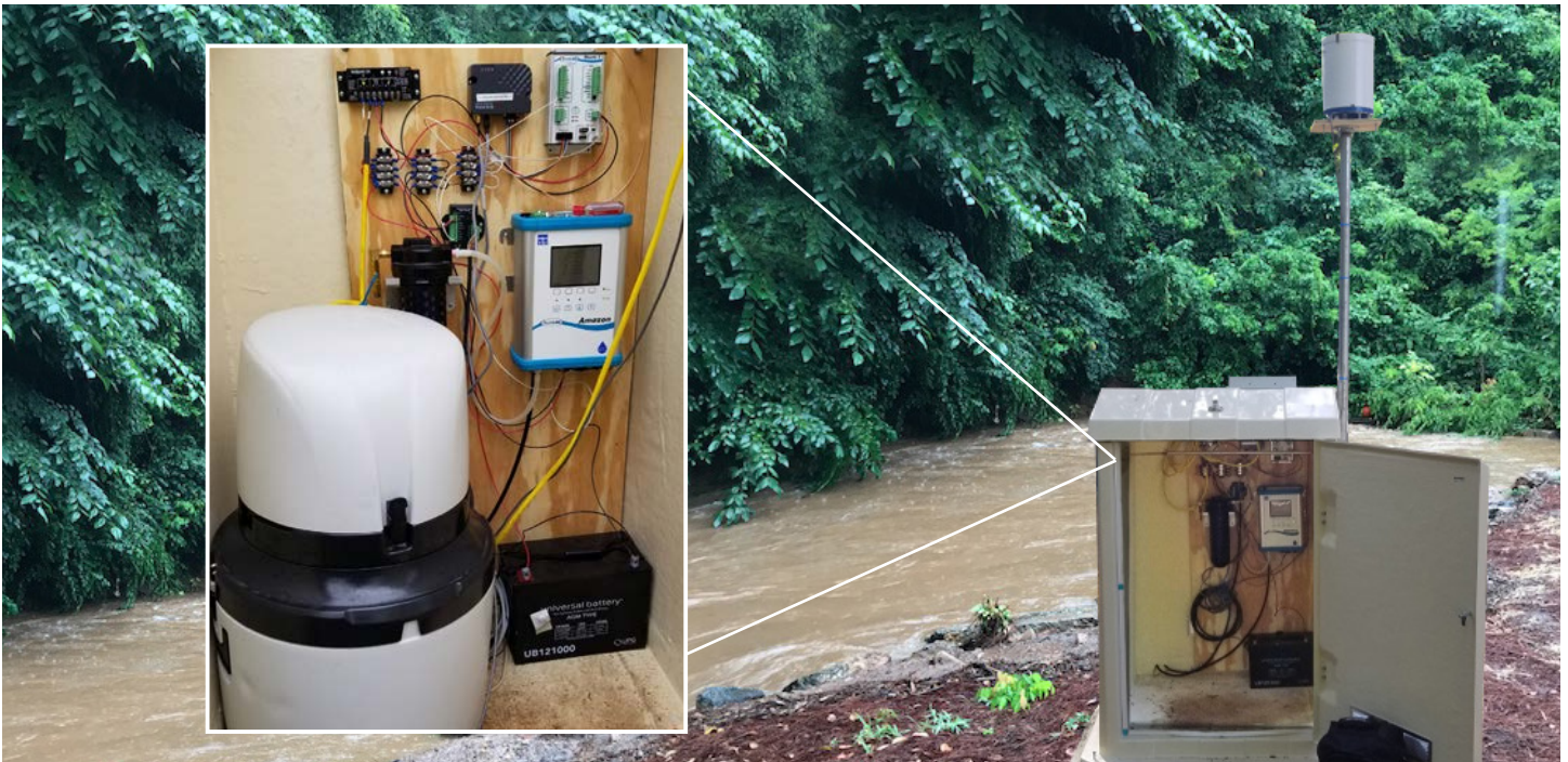
A continuous water monitoring station installed along Tanyard Branch equipped with: an Amazon water level Bubbler and EXO multiparameter water quality sonde, Storm Datalogger, and ProSample sampler.
